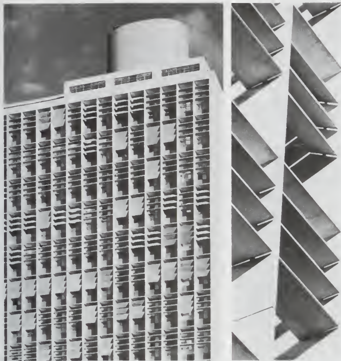
Brise-soleil, shown in (left) exterior and (right) close-up view of the Ministry of Education and Health, Rio de Janeiro, designed by Lúcio Costa and Oscar Niemeyer, 1937–43, Le Corbusier, consultant
